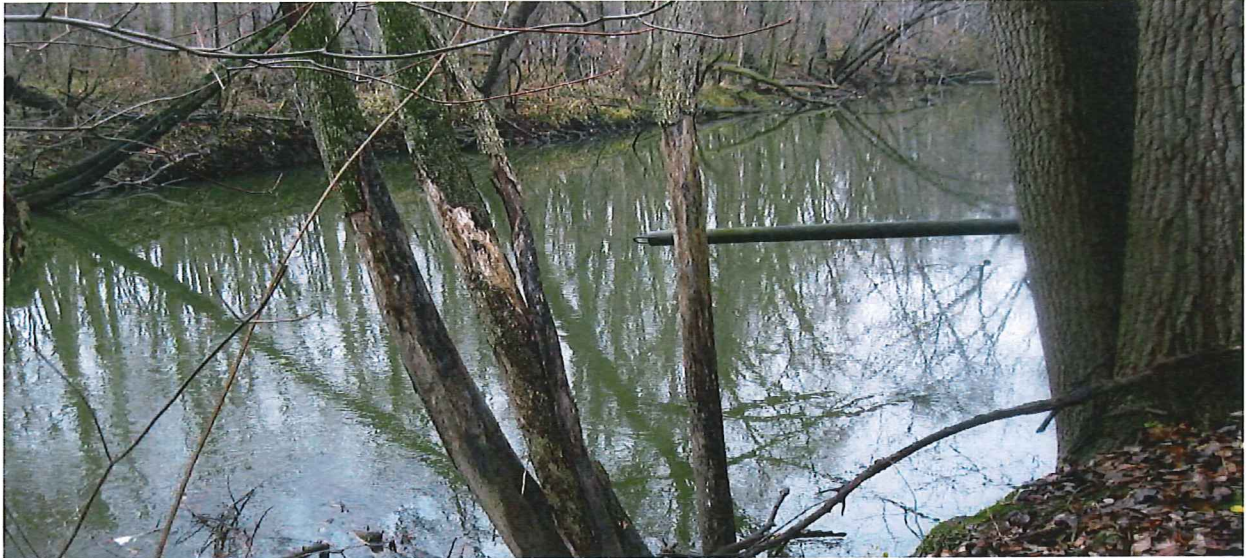
Photo 9 (Section 1 – south bank looking downstream): Pipe from treatment plant overhanging over part of river
