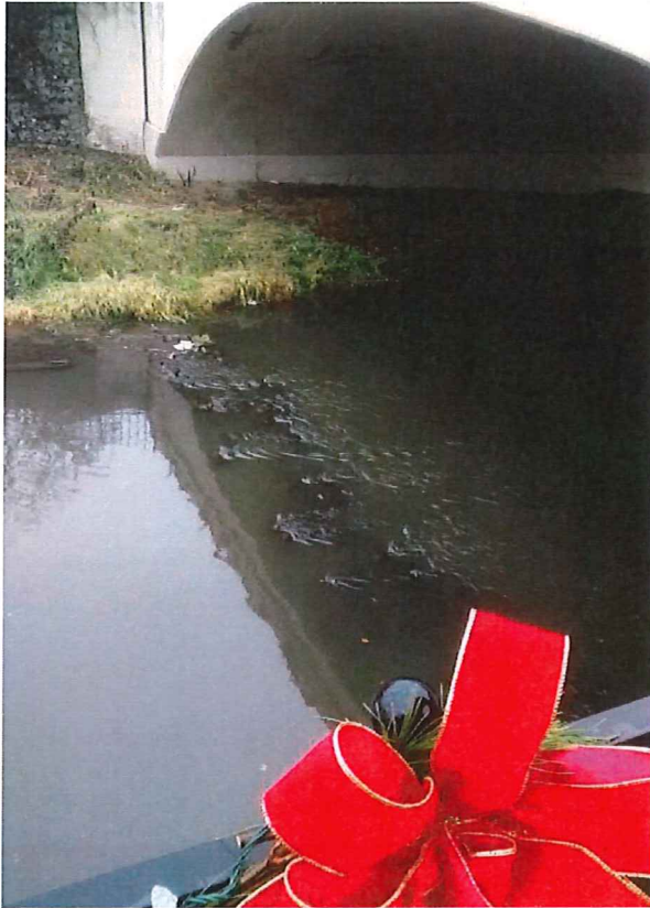
Photo 20 (Section 3 – east bank looking across river under Maumee St. Bridge): Rocks under bridge create shallow conditions in river.
