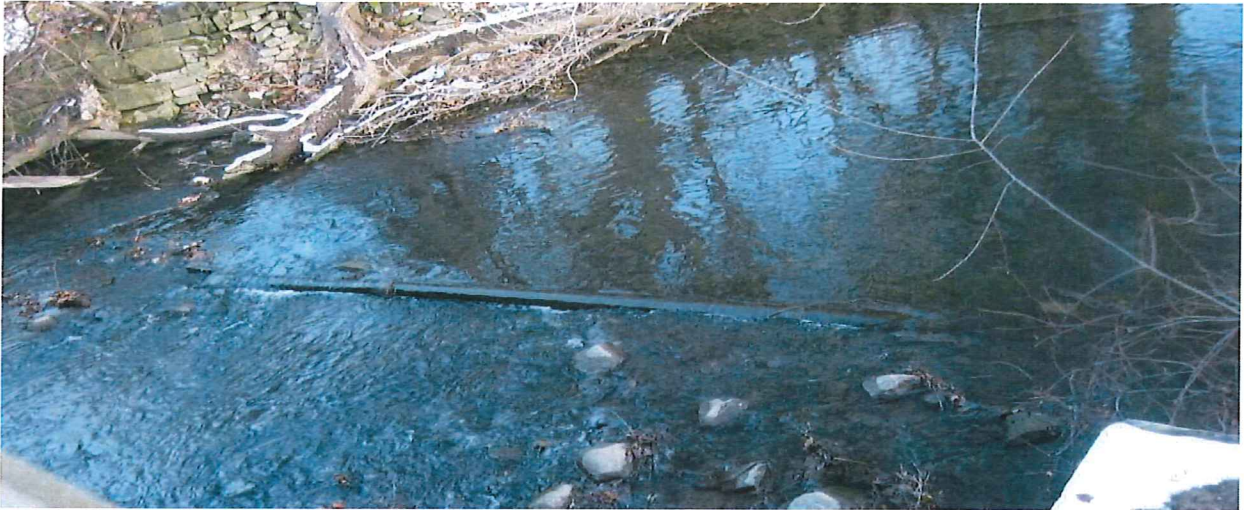
Photo 27 (Section 4 – Looking down from College Avenue Bridge south side): Pipe breaks surface of water
